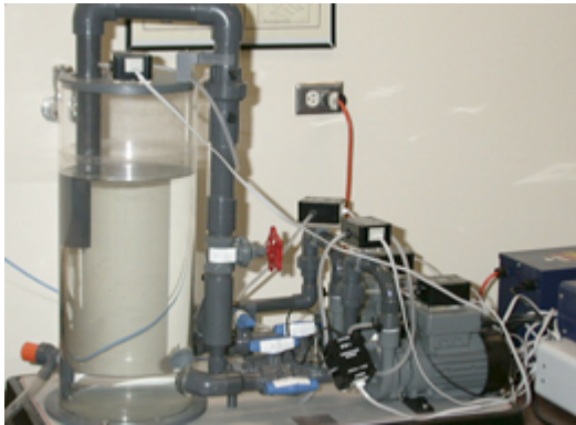
Centrifugal Pump System
